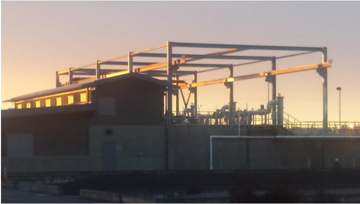
The City's new secondary treatment process MBR went on-line October 2014.
